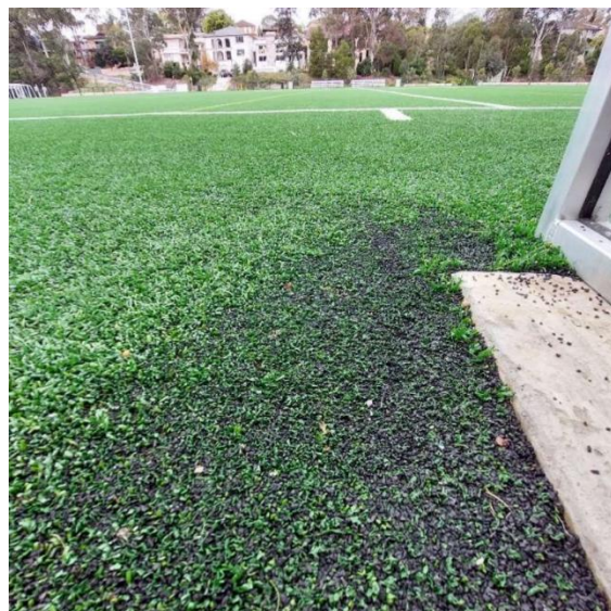
Crumb rubber infill on the synthetic turf playing field at Poulton Park showing the build-up on the edges of the ground.
